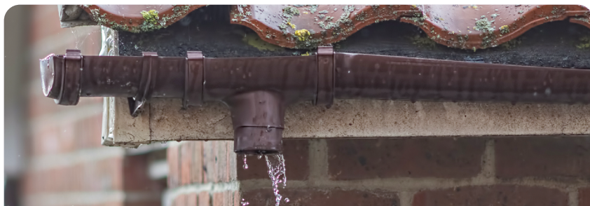
Example of a broken downpipe and gutter leaking water
