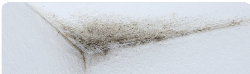
Example of a black mould forming on a ceiling
